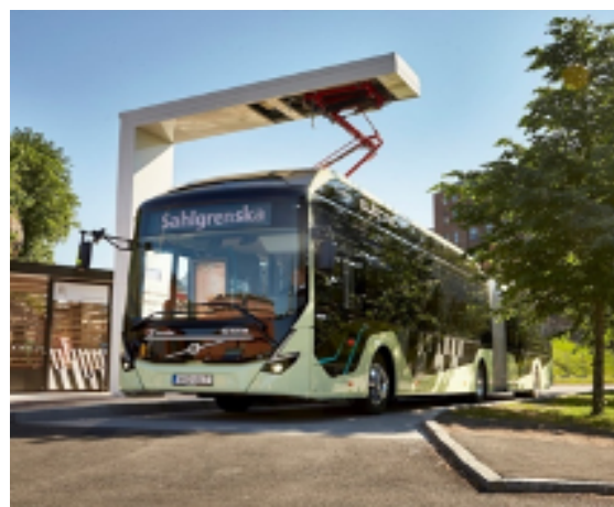
Figure 6 | An e-bus charging through a pantograph
