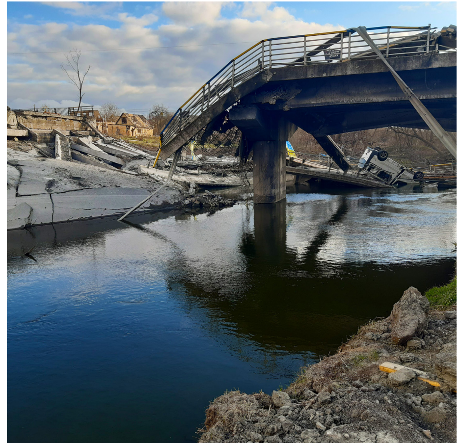
Destroyed bridge in Irpin (Source: CC BY-SA 4.0, https://uk.wikipedia.org )
