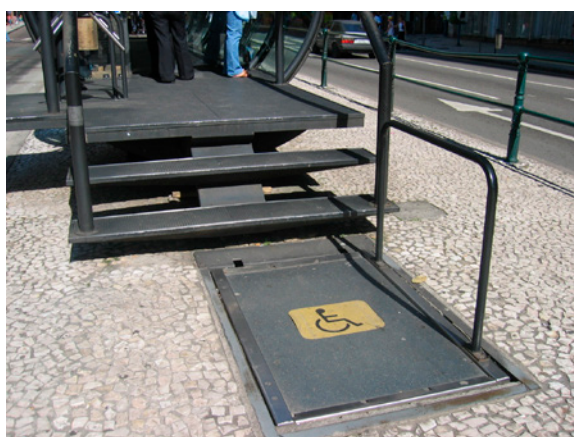
Figure 42: Technical solution for barrier-free access to a BRT station in Curitiba, Brazil. © Karl Otta 2005
