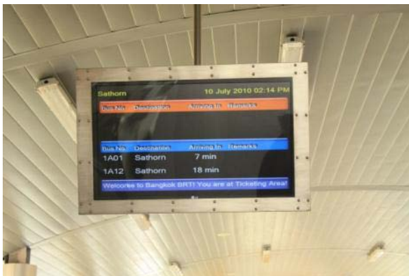
Figure 6: Information system at the BRT Sathorn station
