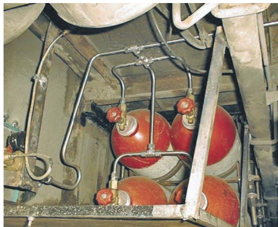
Fig. 3-3 CNG piping in a converted bus, without stress relief loops and inadequate clamping of gas pipes.
