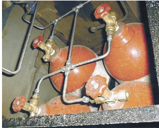
Fig. 3-2 CNG piping in a converted bus, without stress relief loops.
