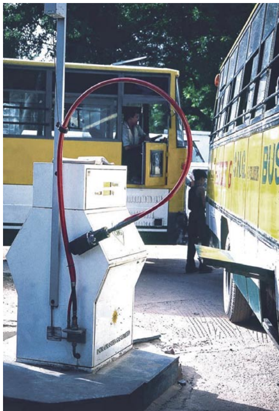
Fig. 3-5 CNG bus refuelling station, Delhi.
