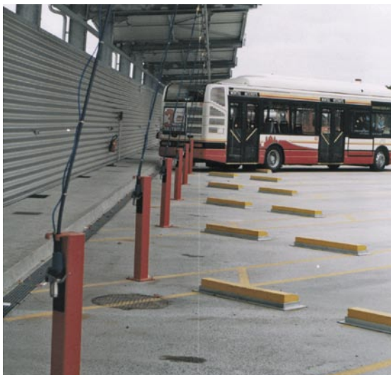
Fig. 2-7 Slow-filling station in Poitiers, France
