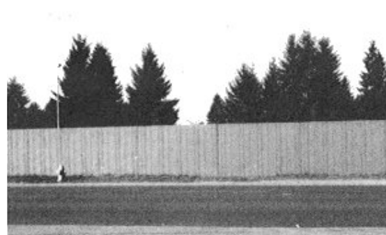
Concrete Noise Barrier with Woodgrain Texture
