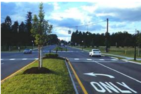
After: The median on the far side is wider to reinforce the left turn lane. Note the bollards to protect pedestrians.
