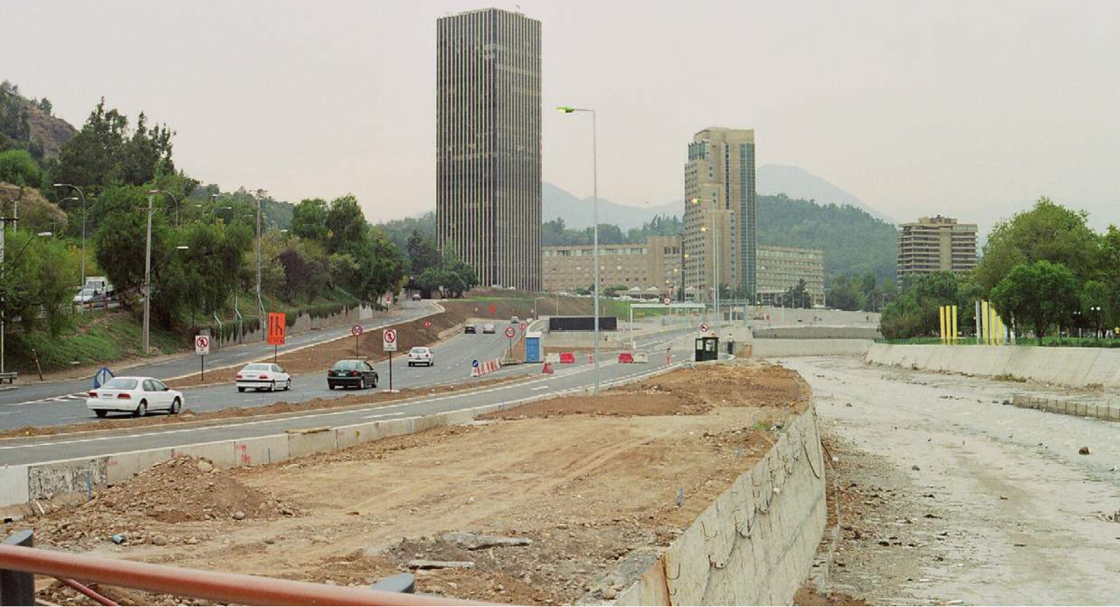
Figure 1. Construction of the autopista Costanera Norte in Santiago, Chile. Photo: Claudio Olivares Medina
